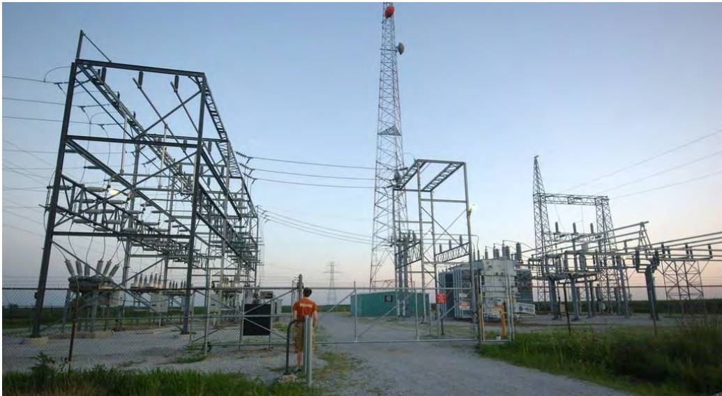
Figure 4. Electric Grid Substation with Microwave Communications Dish on Tower Photo credit: Creative Commons/vaxomatic
